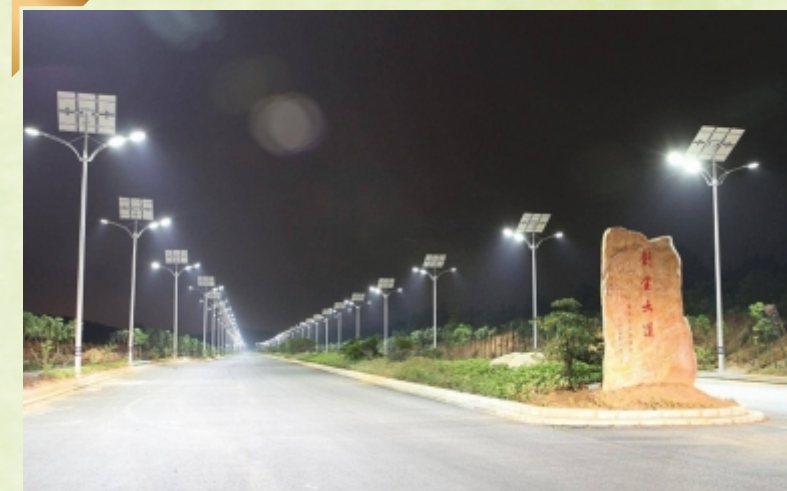
Solar Street Light
